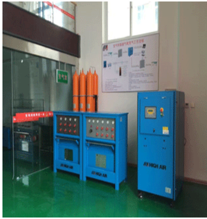
Gas cylinder filling chamber
